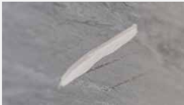
Crack in the elastic upper layer
