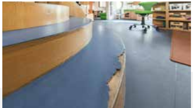
Before: Worn linoleum flooring with patches missing
